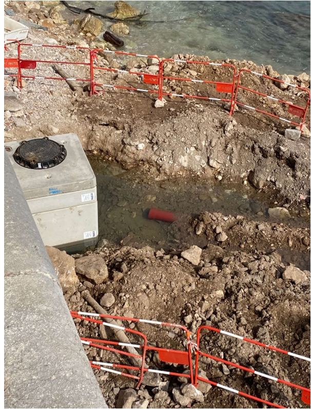
Installation regard provisoire
